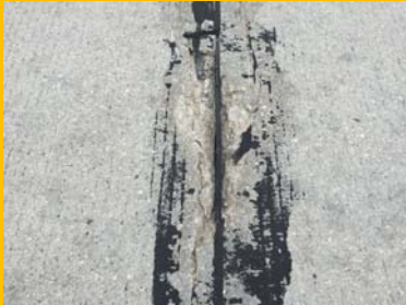
ACR CAUSED THE CONCRETE JOINTS TO EXPLODE!
