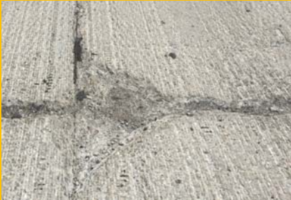
3" MILLING CONCRETE PAVEMENT: DID NOT REMOVE ALL DETERIORATION AFTER MILLING.
